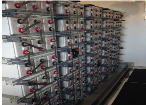
Figure 1: Typical Battery Bank
