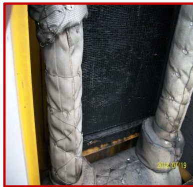
Exhaust with Insulation
