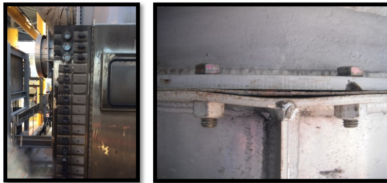
Burn Damage (left), and the Gap in the Mating Flange in One of the Fire Tubes (right)
