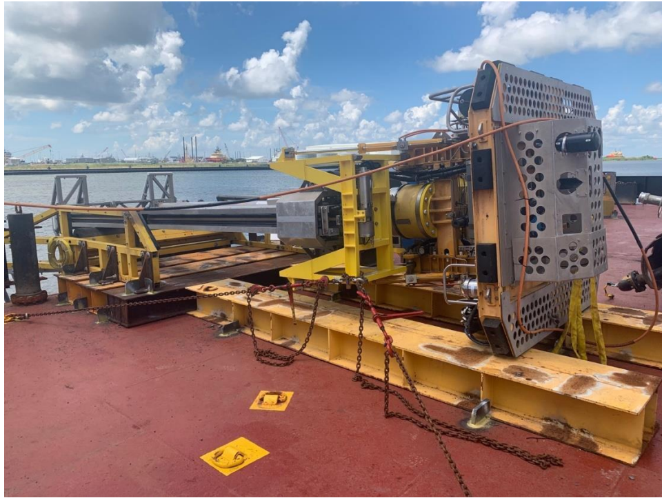
Figure 13 - LARS test fit with AC3. Leg brace omitted and I-beam installed to ensure clearances with stab guide during lift
