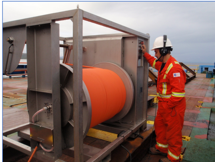
Figure 11: AC Umbilical Winch
