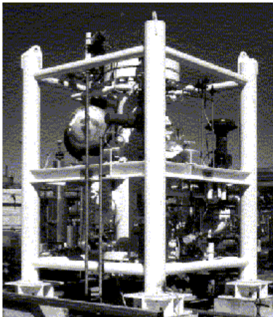
Fig.3.38. Prototype installed in field
