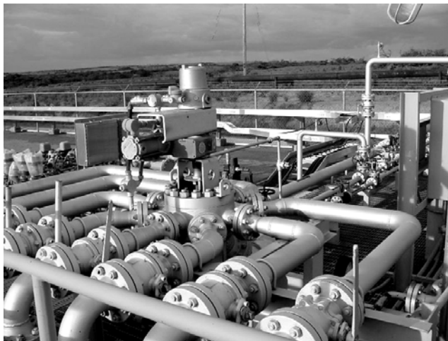
Figure 9.3: A multi-port valve switches production of each well from the main line to the multiphase flow meter.
