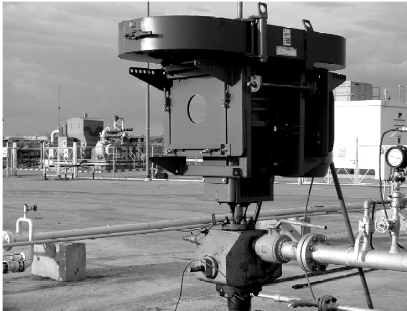
Figure 9.7: This field in a Petrozuata oilfield (Venezuela) combines conventional downhole pumping with surface multiphase pumping.
