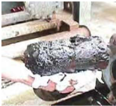
Figure 5.2: An asphaltene plug removed from a pipeline 5 .
