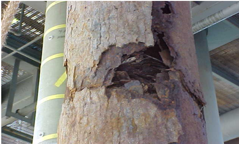
Figure 15.2: Photo of heavily corroded conductor
