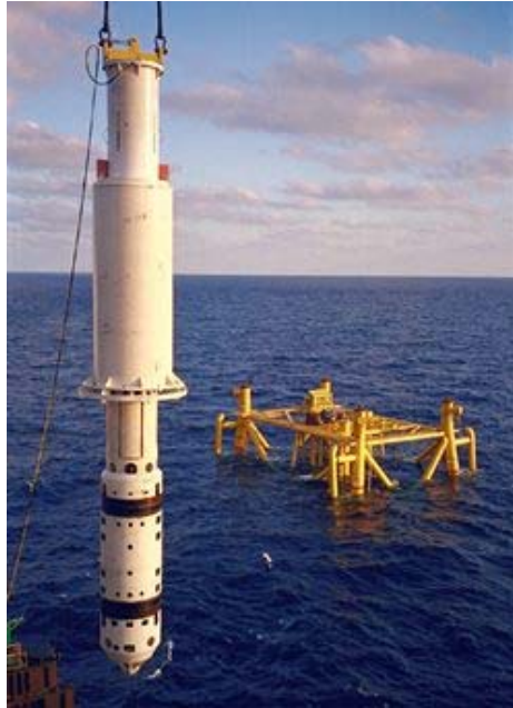
Figure 16.1: An 84-inch Oil State Hydra-Lok tool being deployed to the skirt piles of a jacket in 693 feet (211 m) of water
