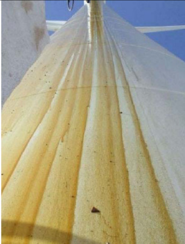
Environmental – Oilspill down the tower from gearbox of wind turbine (Spain)
