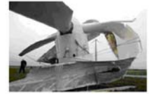
Fig. 18: Structural collapse of a wind turbine in 2002 in a storm. Source: Der Spiegel, DPA.
