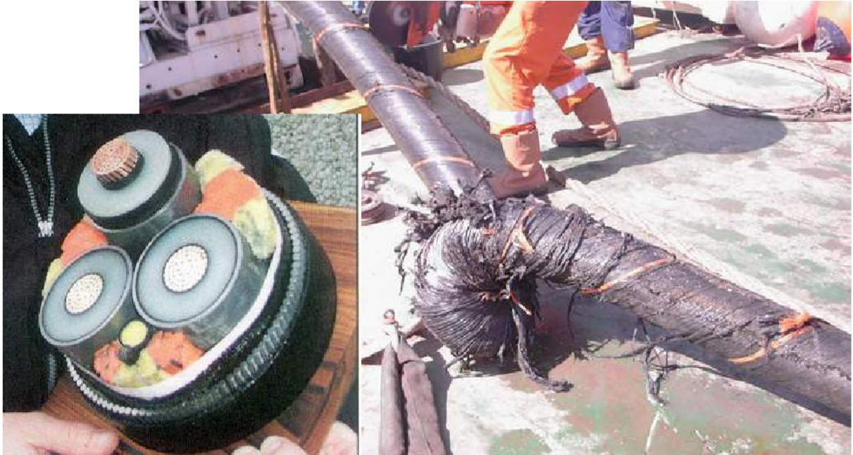
Figure 11: Kinks in Subsea Cables
