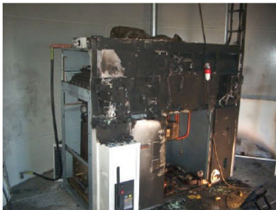
Short circuit in a power panel. Root cause was a bad connection on a high power cable.
