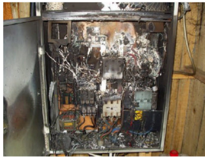
Short circuit in a power panel. Root cause was lightning.
