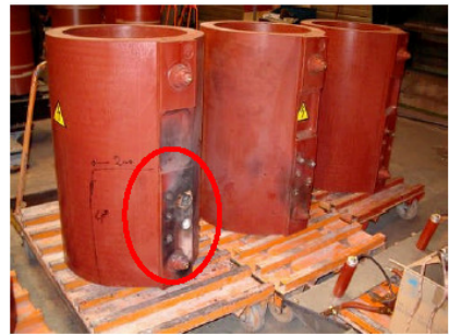
Short circuit in the transformer. Root cause was probably high temperature due to insufficient cooling.
