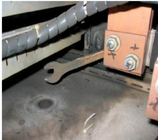
Short circuit in a power panel. Root cause was a forgotten tool. It was traced back to the manufacturer.
