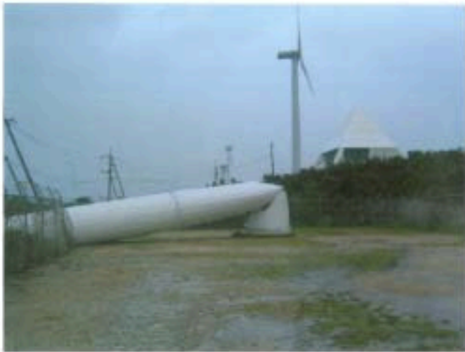
Fig. 1 Buckling Failure of a Wind Turbine Due to Typhoon C20030911.1f.psd
