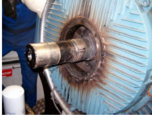
Hot bearing from a 1 MW generator. Root cause could among others be lack of grease, unsuitable grease or loose connection between bearing and shaft.
