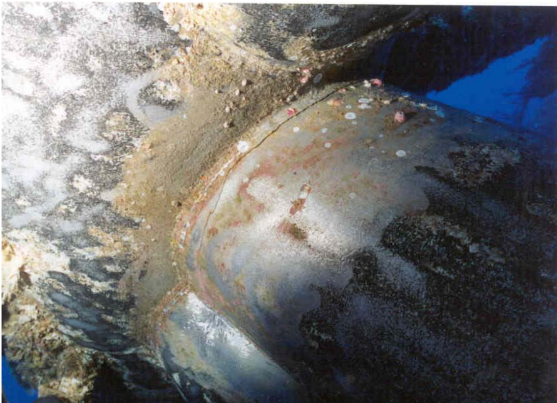
SS 291 A, Close up of the 360° Crack at the B2 Leg
