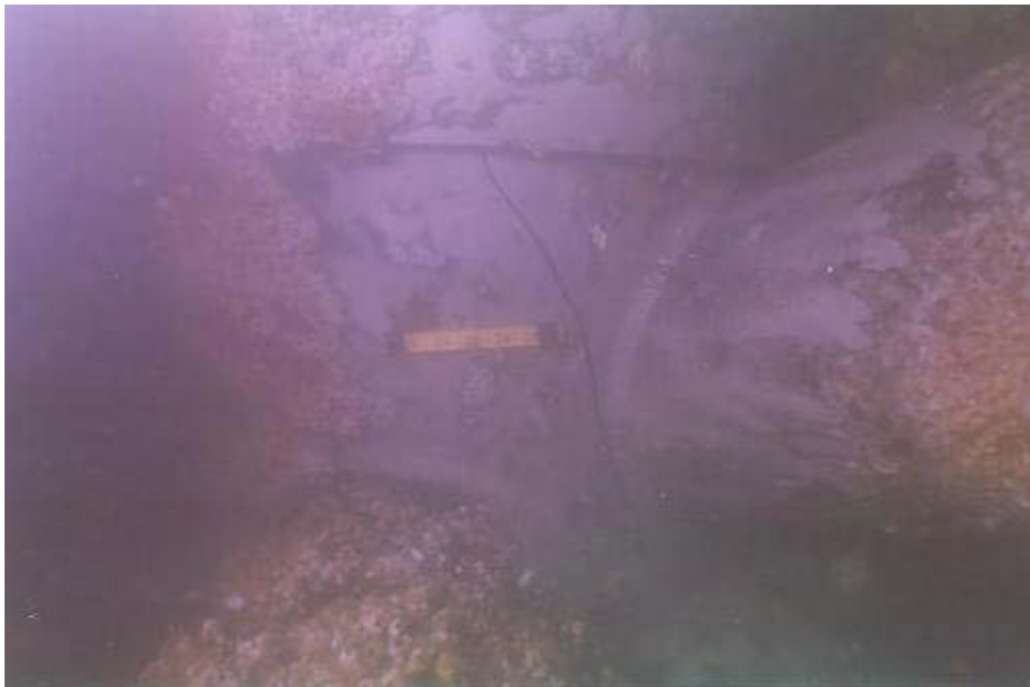
Ship Shoal 169 A – Crack Propagation Beneath Riser Clamp
