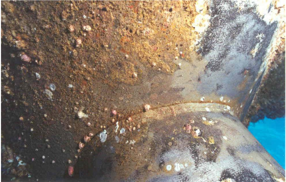
SS 291 A, Close up of the 360° Crack at the A2 Leg
