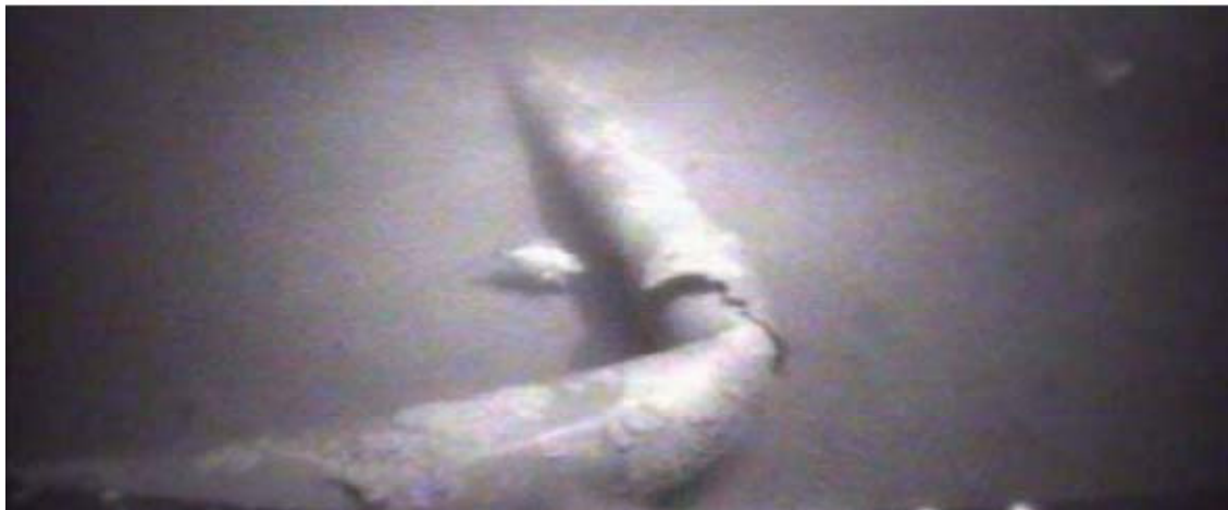
Figure II.7: Kinked Pipeline Hurricane Damage
