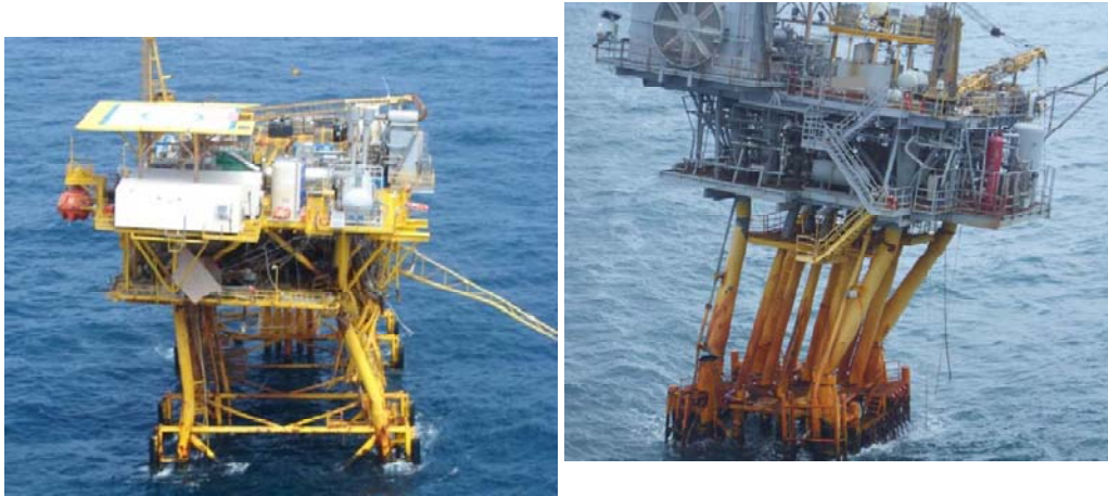
Figure VI.6: Wave-in Deck (WID) Damage to GOM platforms from Hurricane Ike 2008
