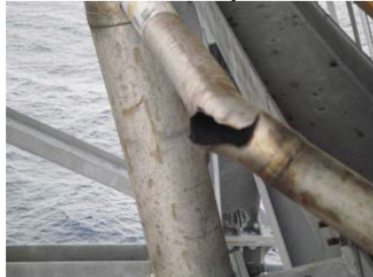
Ruptured Interconnected Pipe
