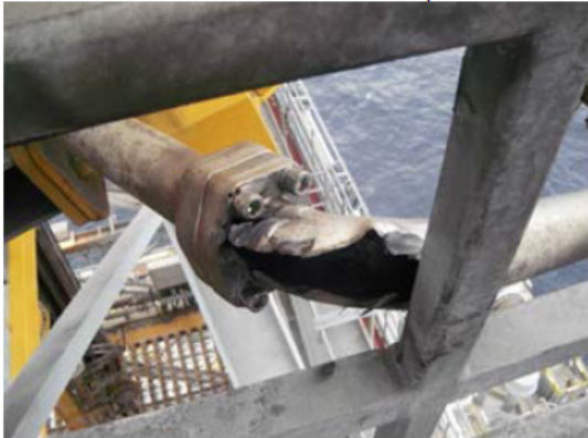
Ruptured Interconnected Pipe
