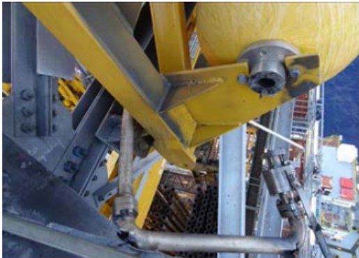
Failed CAPV and Interconnected Pipe
