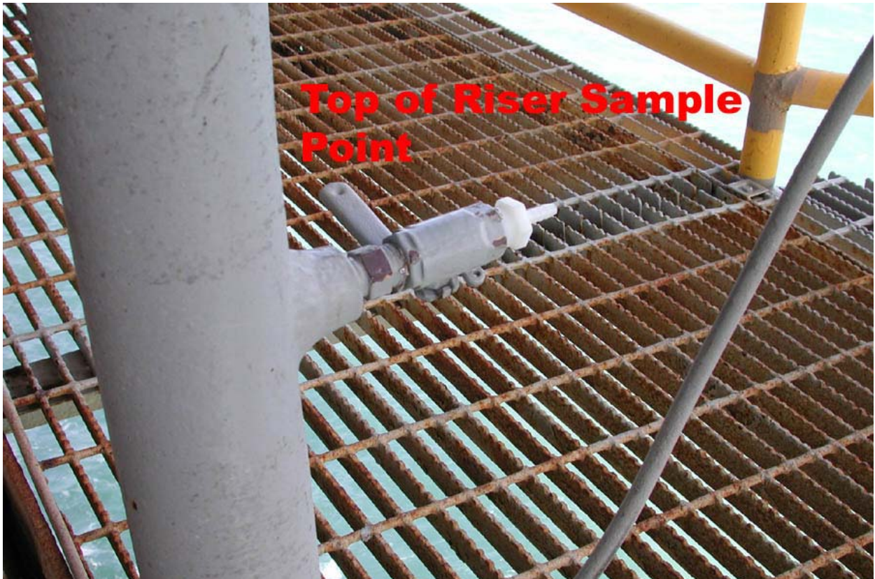
This photo shows a typical top-of-riser sample point at the receiving platform.
