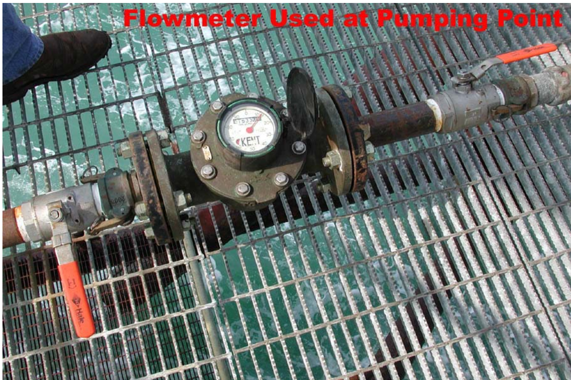
Photo #1 The flowmeter reads in hundreds of gallons pumped. It was “zeroed” and calibrated prior to commencing work.
