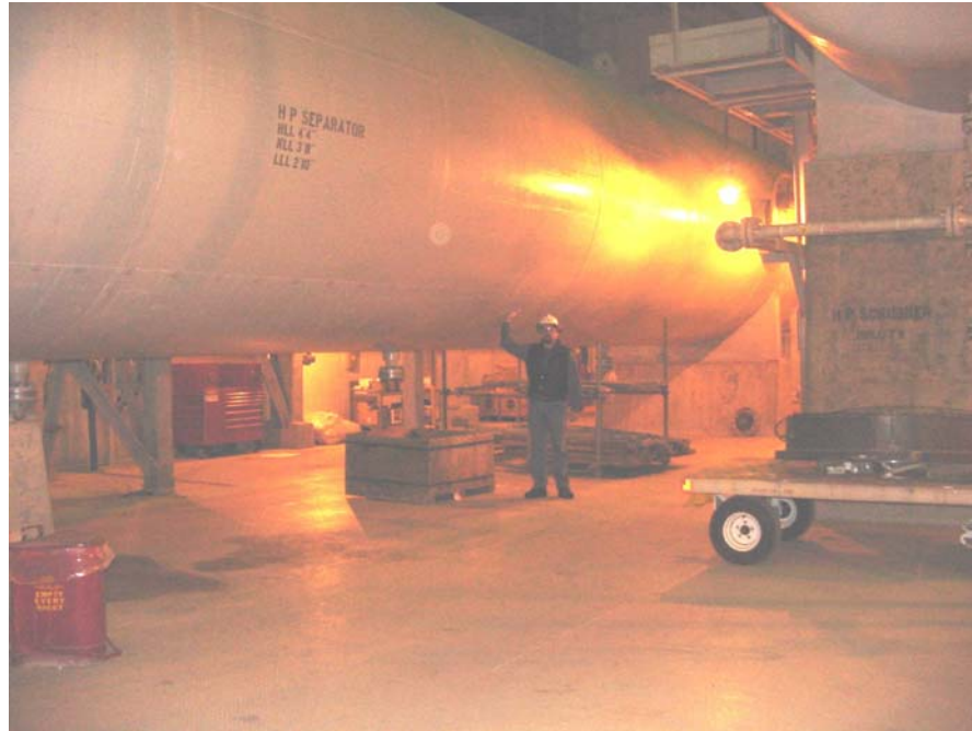
Figure 5.7: High Pressure Separator - Prudhoe Bay Field, Alaska
